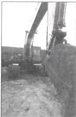
Heavy equipment was used to install over 2000 feet of 12 inch sewage pipe.
