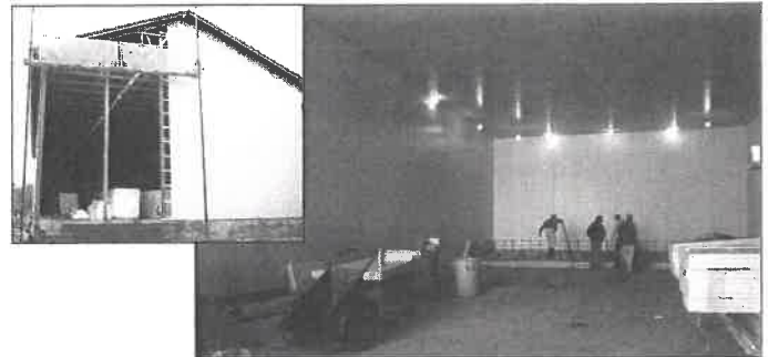
Romeo's expansion will add 4,000 sq. ft. of new refrigeration space to its present facility.
